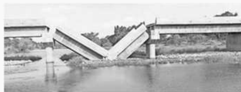
A newly built bridge on Mindhola River collapsed in Tapi in June.
